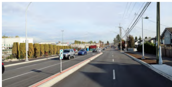
A section of 80 Avenue that was widened to four lanes in 2023. Surrey Council has approved a contract to continue this road improvement and widening project to extend all the way to King George Boulevard.
